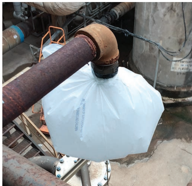
FIG. 5. Trash bag test on the after-condenser vent to measure the total non-condensable load from the surface condenser and inter-after condenser units.
