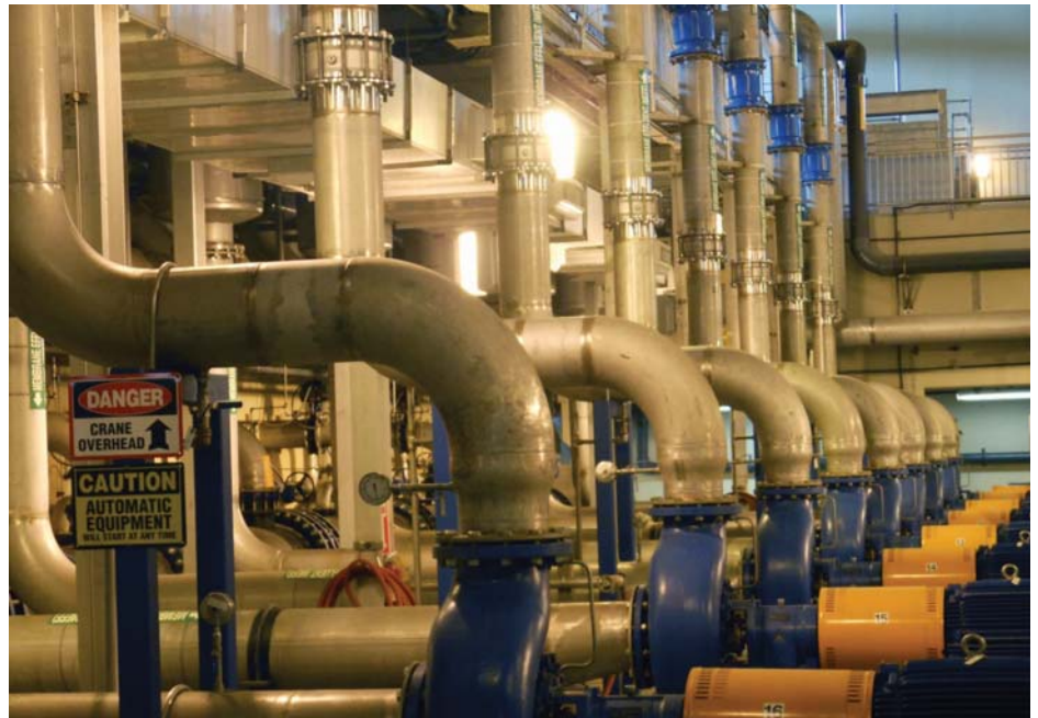
The current installation updated with DFT axial flow check valves installed in a vertical flow up orientation, eliminating the hydraulic shock/water hammer in the membrane facility.
